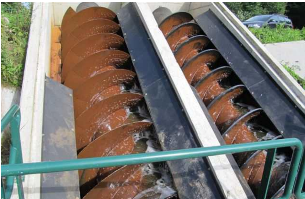
Figure 2.2 Pumping station at Ennemaborgh with screw pump 1 (left) and screw pump 2 (right).
